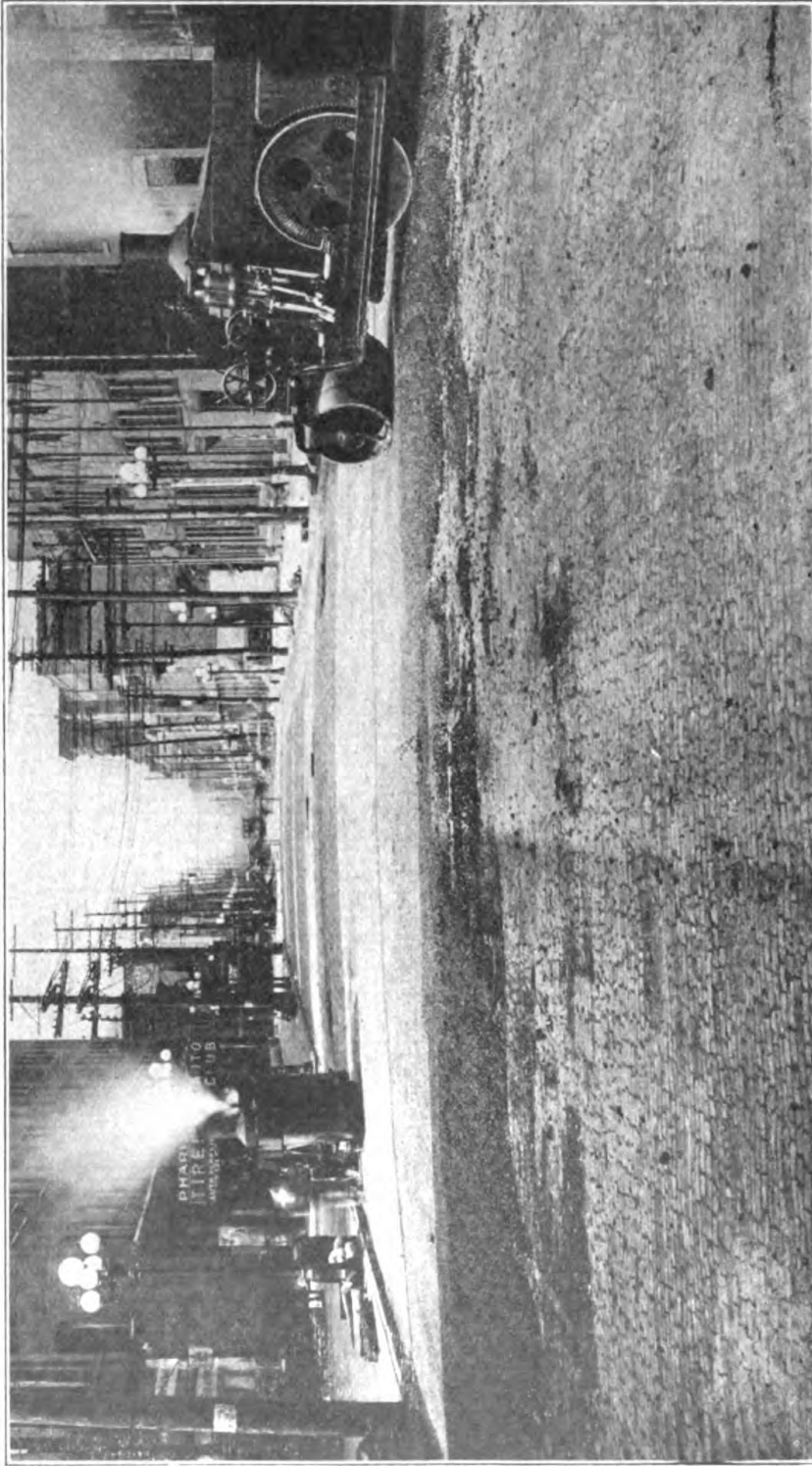
Resurfacing old brick pavement with asphalt, using binder coat and wearing surface coat. Asphalt laid from curb to curb. Gay Street, between High and Fifth Streets, Columbus, Ohio, 1912.
